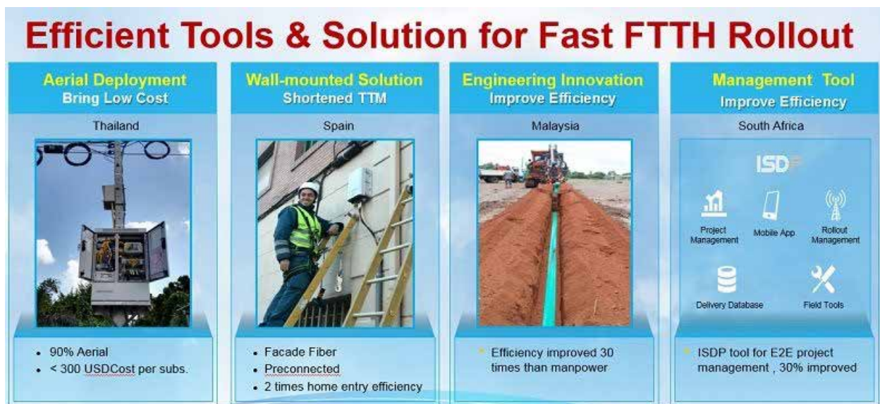
FIGURE 3. Several advances can speed the deployment and reduce the costs of all-fiber gigabit broadband networks.
